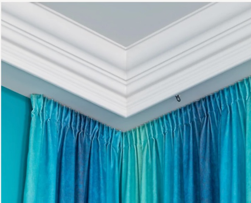
Noël & Marquet decorative profiles at the Nuvole Garden Hotel di Brunate - Ph. Credits Noël & Marquet
